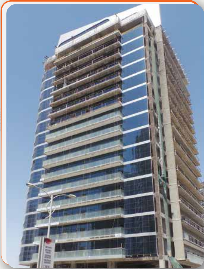
OASIS TOWER I 2B + G + M + 18 + FLOOR PLOT NO. 682-125 FOR FAKRUDDIN FACILITIES MANAGEMENT
